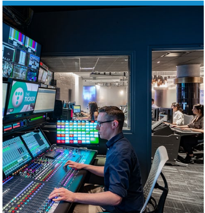
Top of front page: The configuration of the Reception Hub and Control Room 1 at Verizon Media was carefully considered to balance contrasting work environments. Above: Each control room at Verizon Media has a dedicated audio booth providing multiple positions with visual connectivity to the control room and Reception Hub beyond. Photos: © Adrian Wilson.
